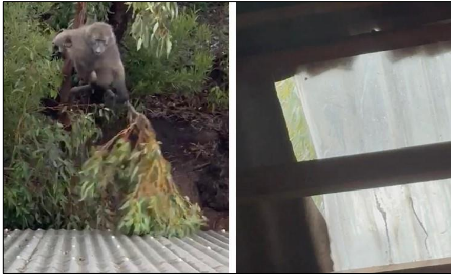
Figure 15. Baboon accessing Heron Park via overhanging branches. This leads to roof sheet damage.
